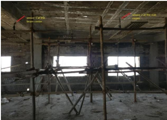
Fig.3. On-site picture of sensors location
