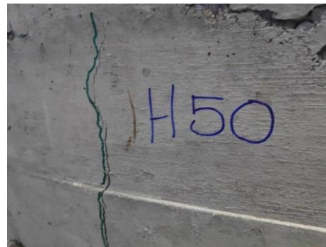
Fig.7. Failure modes of H1 (50mm)
